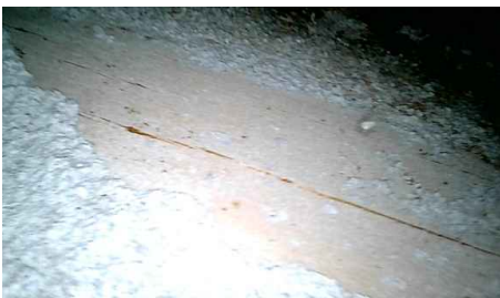
Moisture coming through
