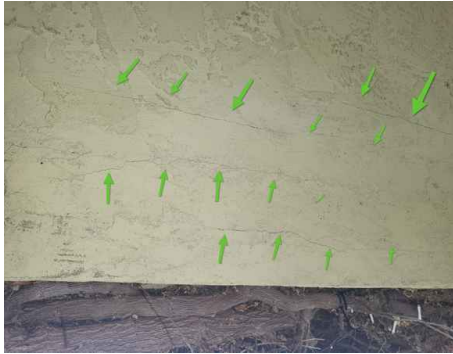
Cracks in stucco soffit
