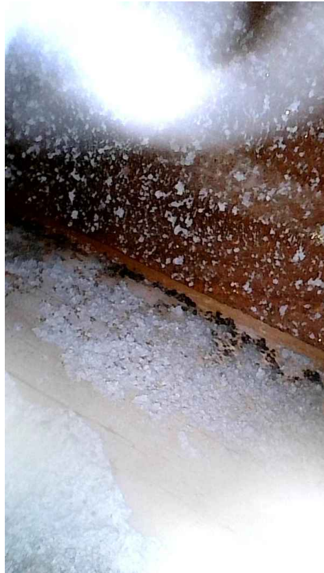
Photo# 8 Termite droppings along rim board
