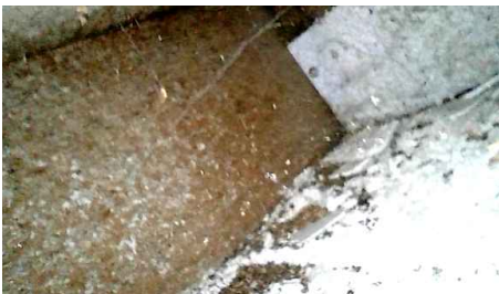
Photo# 10 Termite droppings along rim board
