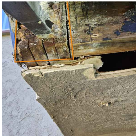
rotten joist, substandard construction
