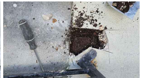
corroded railing connection
