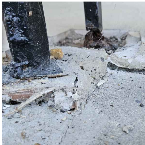
corroded railing connection
