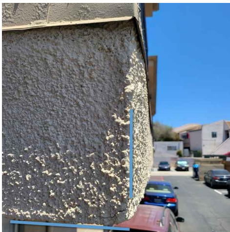
Cracking and puffing
