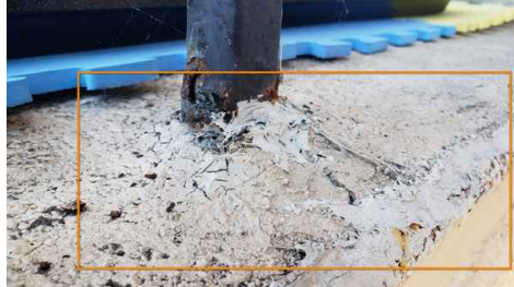
expansion from corrosion
