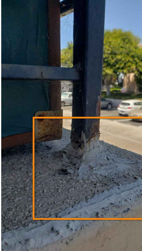
expansion from corrosion
