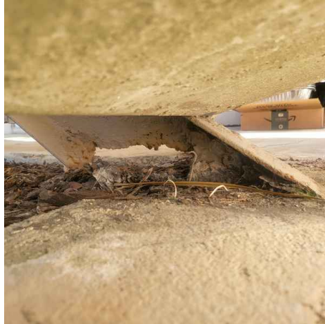
Stringer bottom rusted through
