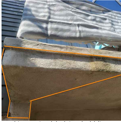
cracking, stained, bulging, bubbling, efflorescing, mold and mildew
