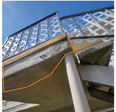
cracking, stained, bulging, bubbling, blistered efflorescing
