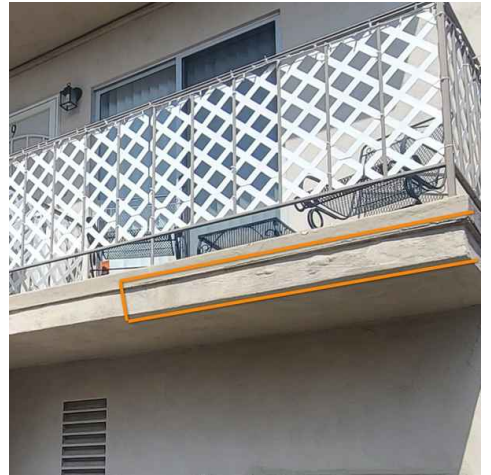
cracking, stained, bulging, bubbling, efflorescing
