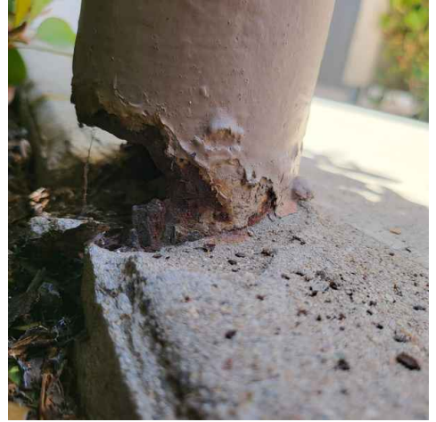
Support post rusted through
