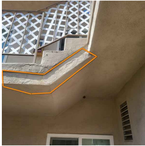
cracking, stained, bulging, bubbling, blistered, efflorescing
