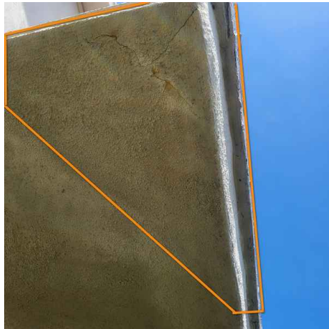
cracking, stained, bulging, bubbling
