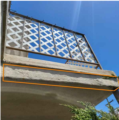
cracking, stained, bulging, bubbling, efflorescing
