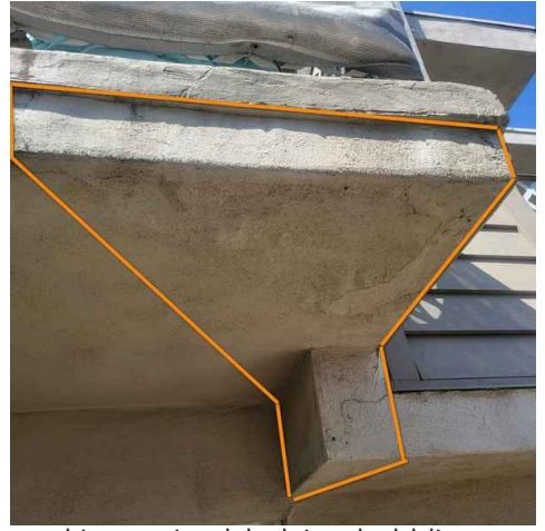
cracking, stained, bulging, bubbling, efflorescing
