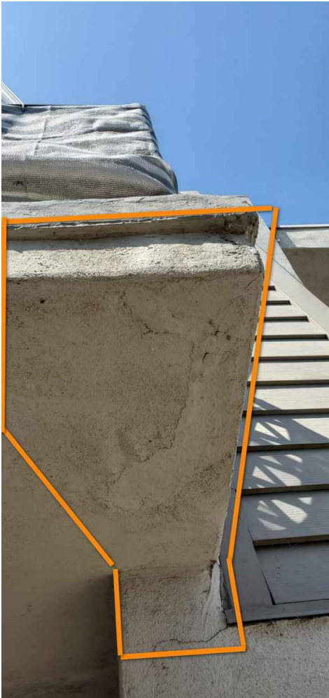
cracking, stained, bulging, bubbling, efflorescing
