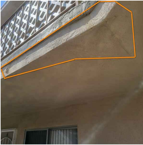
cracking, stained, bulging, bubbling, blistered, efflorescing
