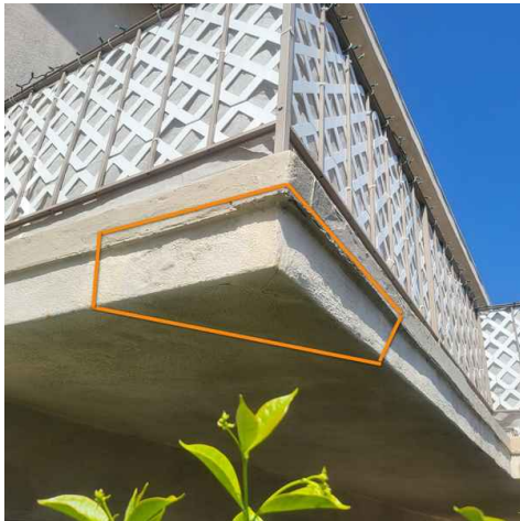
cracking, stained, bulging, bubbling
