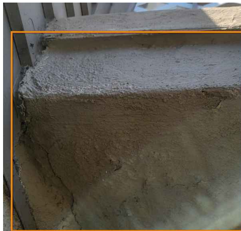
bubbling, efflorescence, blistered
