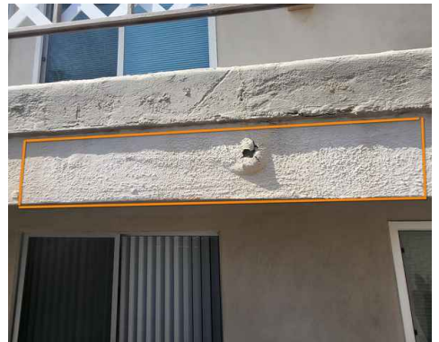
bulging, bubbling, blistered, efflorescing
