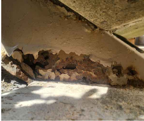
Stringer bottom rusted through
