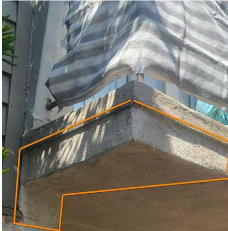
cracking, stained, bulging, bubbling, efflorescing
