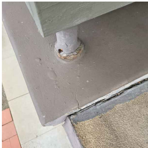
Crack in sealant above termite damage
