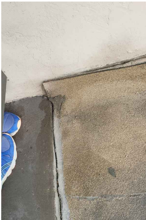
Crack in sealant above termite damage
