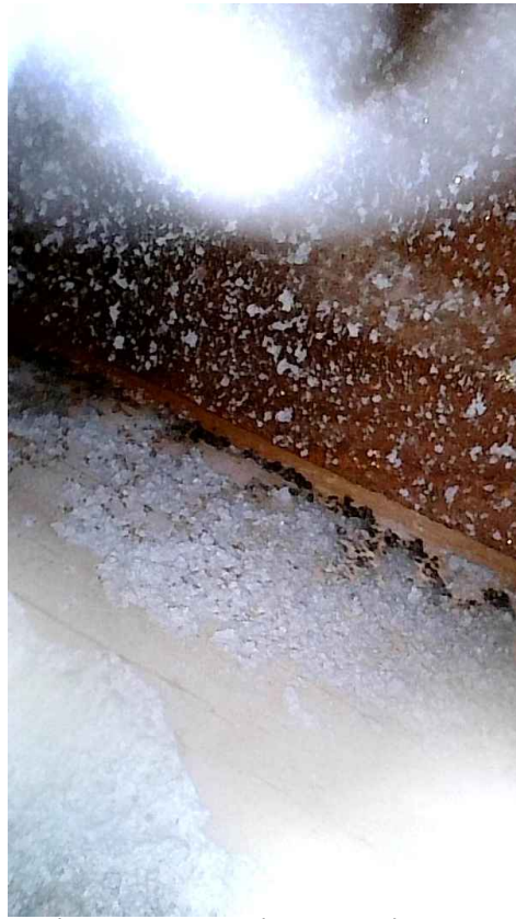
Photo# 8 Termite droppings along rim board
