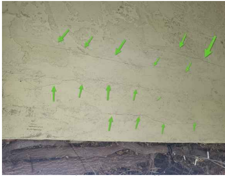
Cracks in stucco soffit
