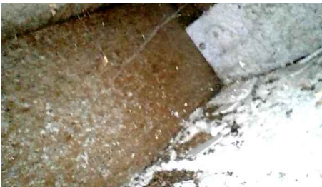
Photo# 10 Termite droppings along rim board
