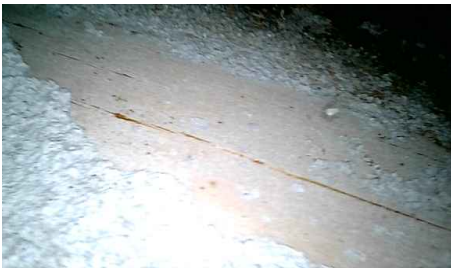
Moisture coming through
