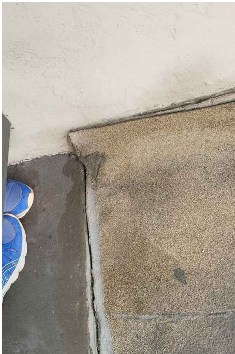
Crack in sealant above termite damage
