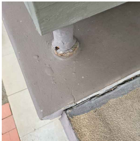
Crack in sealant above termite damage
