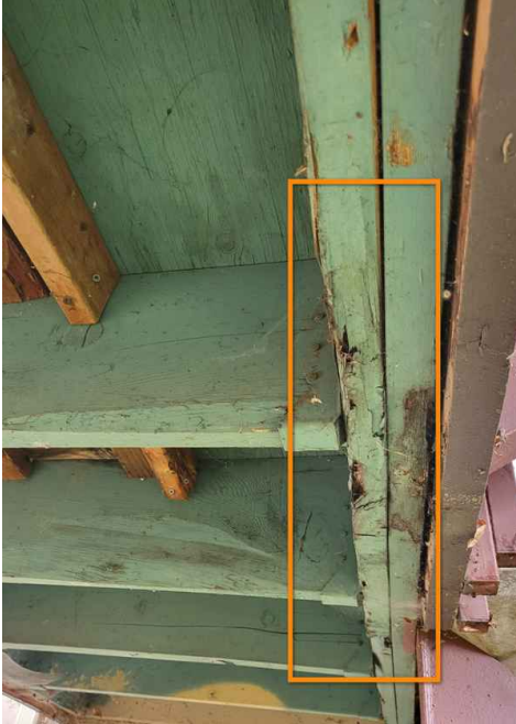
Doubler with Termite Damage
