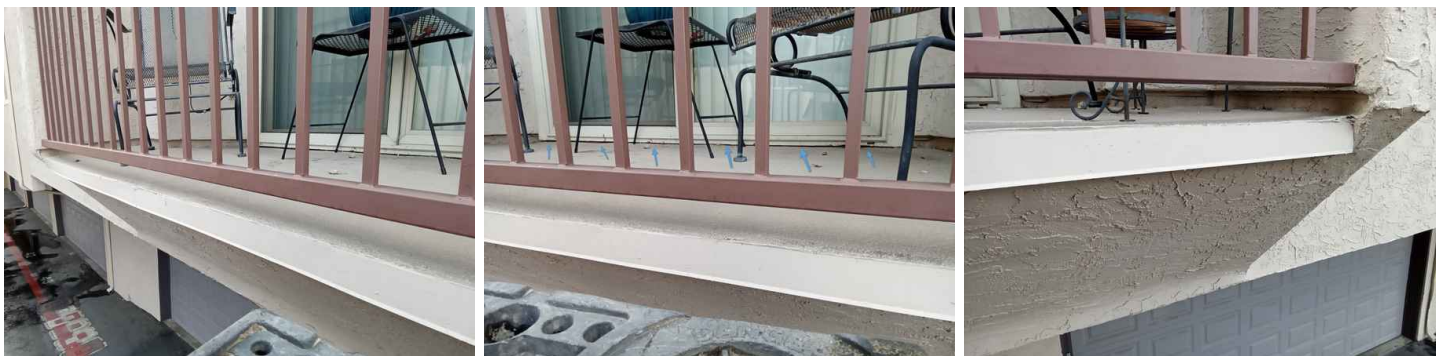
Gap Under Threshold
