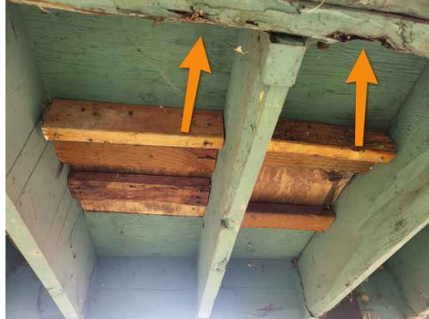
Doubler with Termite Damage
