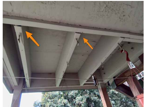
Landing Joist Hangers
