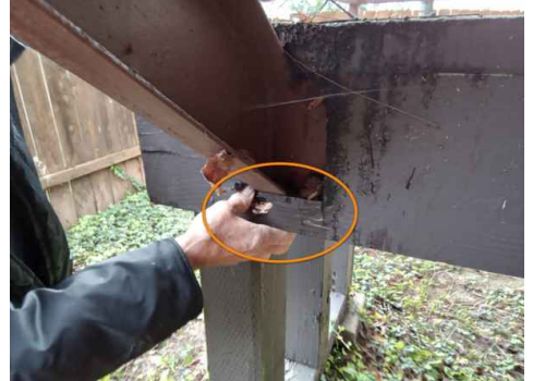
Dry Rot/ Termite Damage
