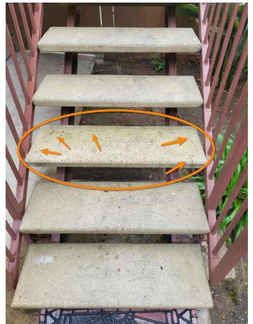
Damaged Stair Tread
