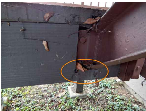
Dry Rot/ Termite Damage
